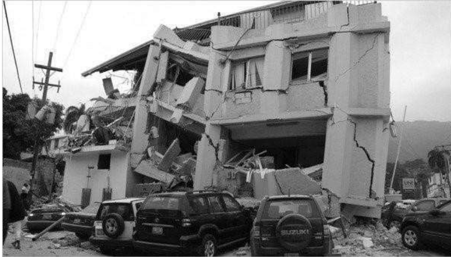
Fig.1.2: Failure of an URM building during 2010 Haiti earthquake
