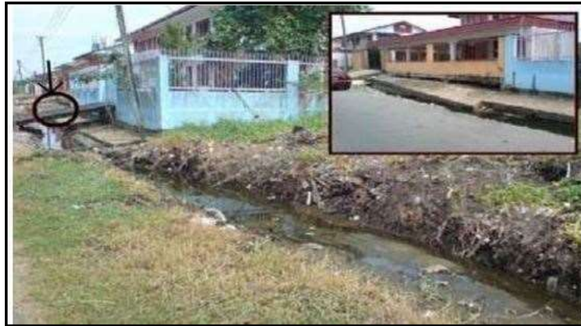
Figure 3: Settlement of peat soil in residential area
